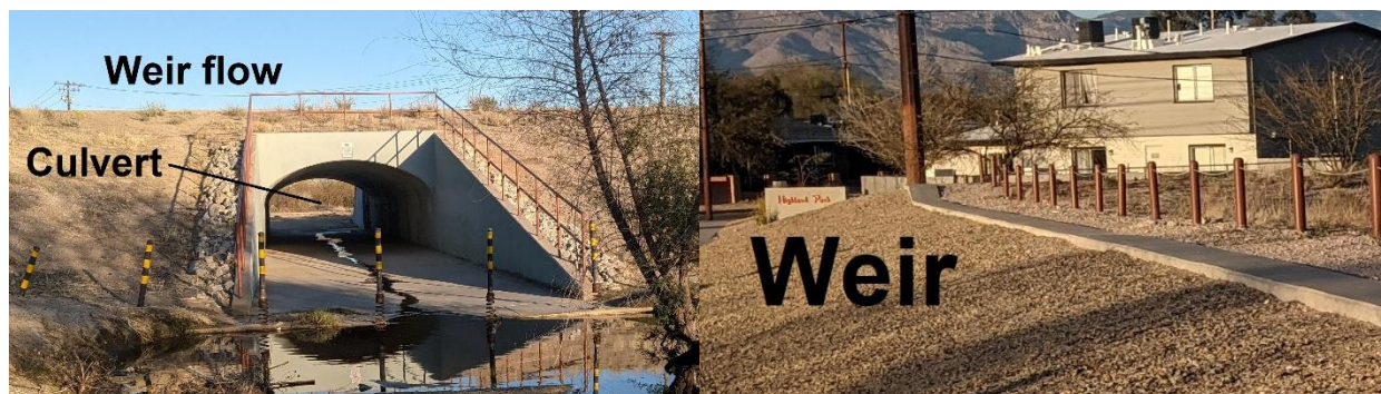
Figure 9. Different flow conditions present in typical detention pond hydraulic structures, at the left an arch concrete box shaped culvert, at the right a detailed view of the weir above the culvert.
